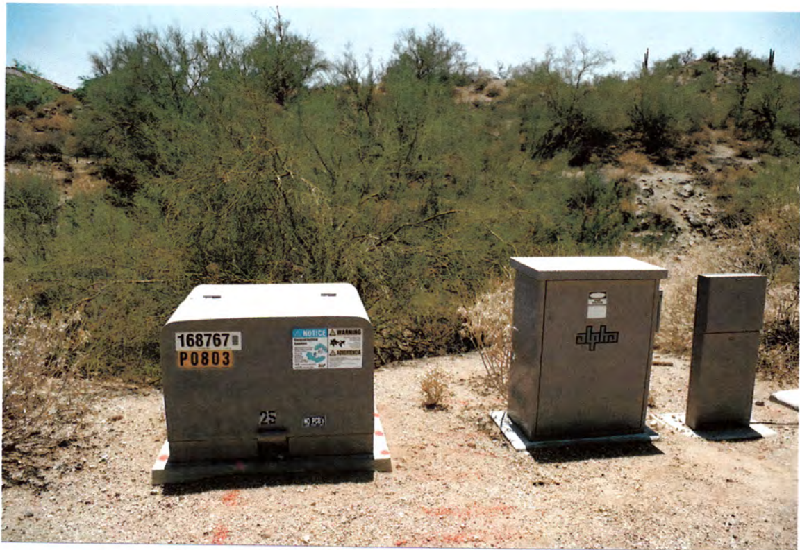
Photograph #2 - View of transformer labeled "tested for PCBs" located at west vicinity-
